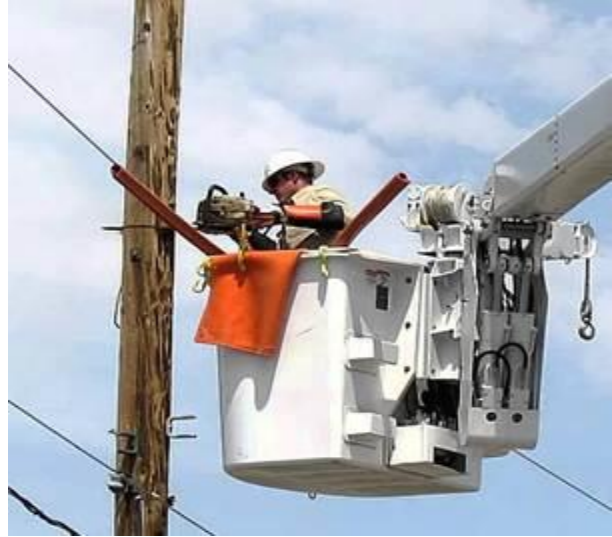
The Solar PV are nearing completion due to this weeks' pole work
