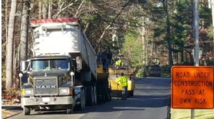
Our Highway Department worked with a contractor to finish paving Pine Street.
