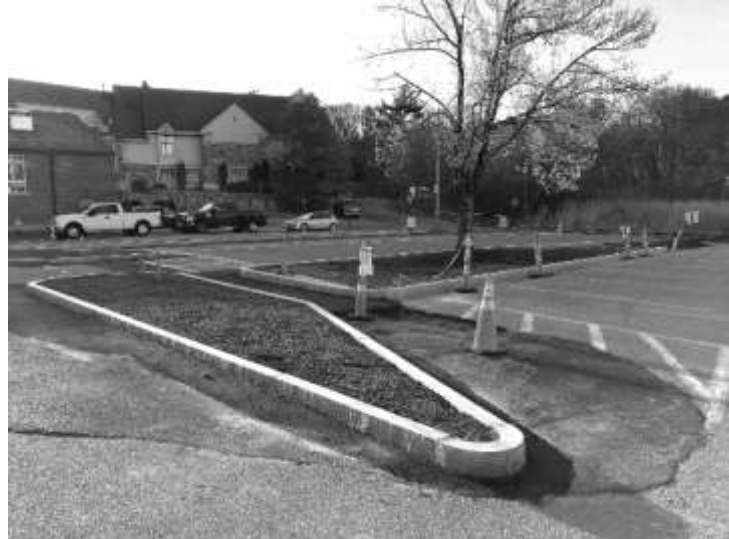
New parking delineations along Center Street as part of the Town Center Improvement Project
