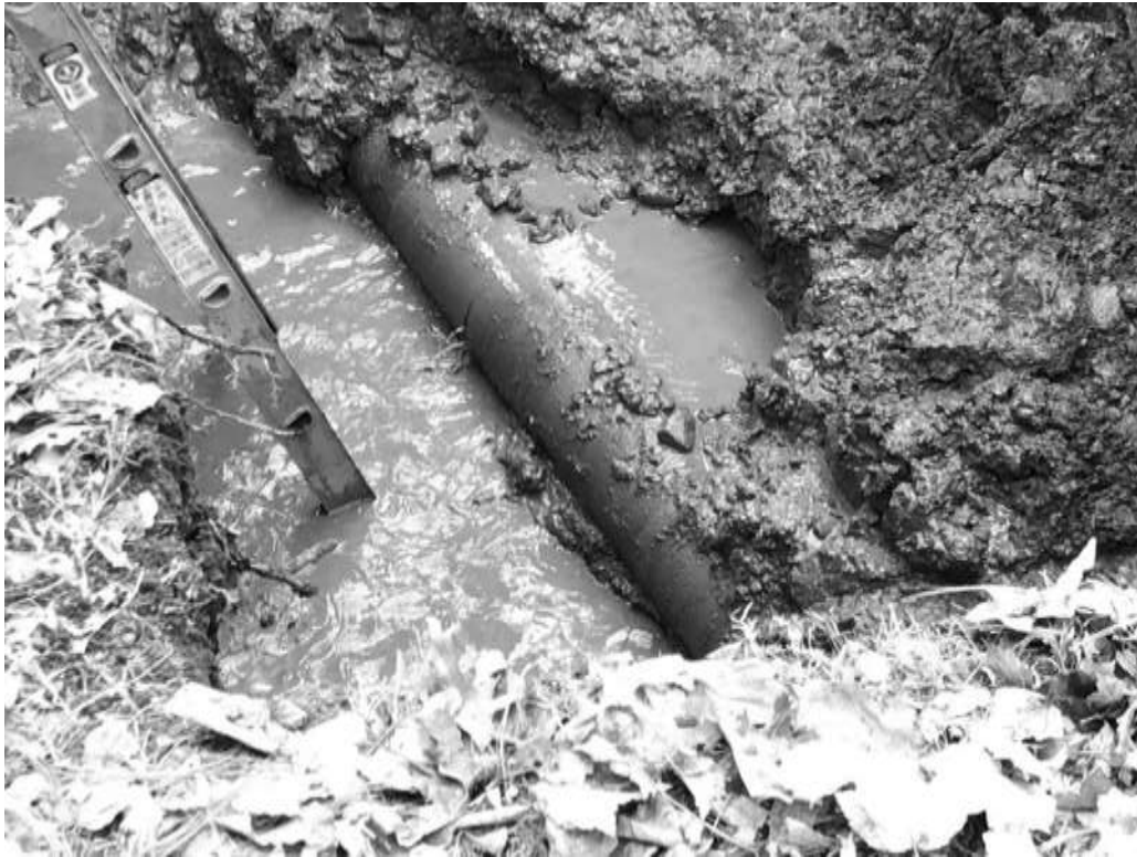
Water Division responded to a watermain break in February on Wood Ridge Road
