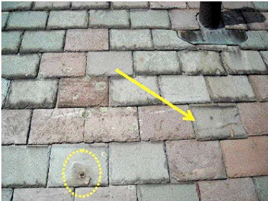
117 year old slate on Building A - deterioration and lichen growth; hole in slate and slates have loosened
