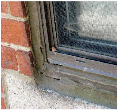
Cracking and splitting of exterior sealant to mitigate water intrusion
