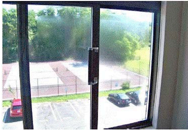
Condensation on the interior of the double glazing caused by a broken gasket
